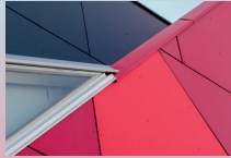
Joints around facade panels
